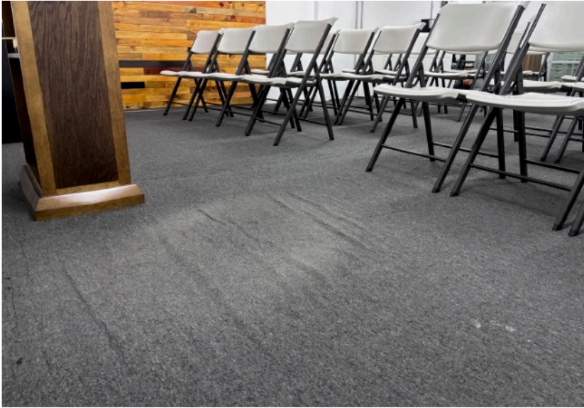
LEFT The building owner estimates the carpet had not been replaced in the last 10 years.
